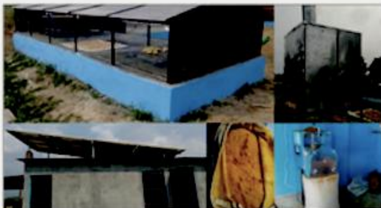
A microgrid powering a food processing unit
