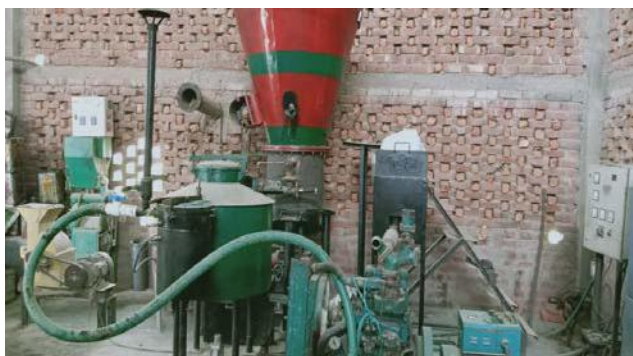
Figure 2. Biomass Gasifier Power Plant at Chakai village
