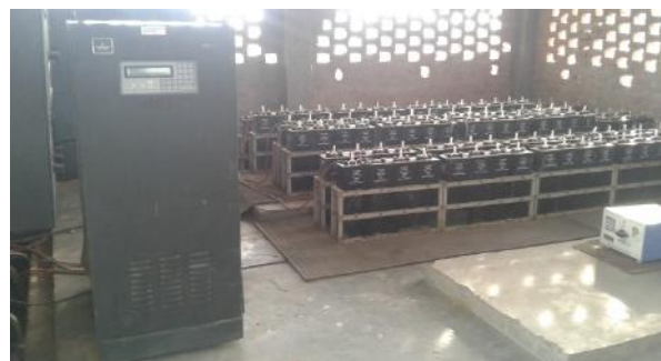
Figure 4. Solar inverter and batteries at Chakai plant
